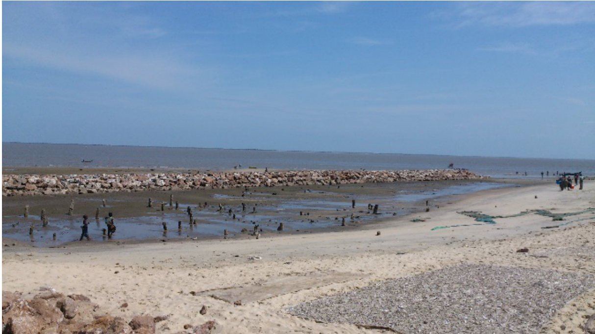
Figure 66: Construction of a new Seawall in February 2013, Praia Nova. Acquired from Palalane et al. (2015).
